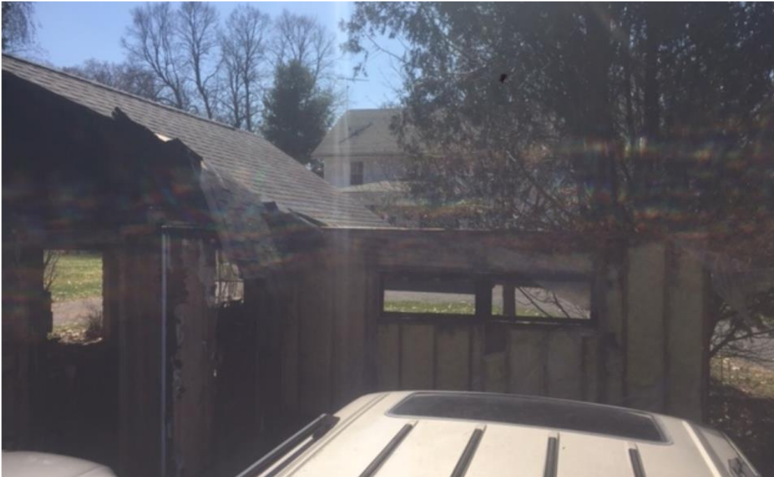
Photo of former garage, largely destroyed by fire.
